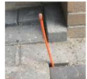
FTTH Connection waiting to be connected to a home in the Netherlands
